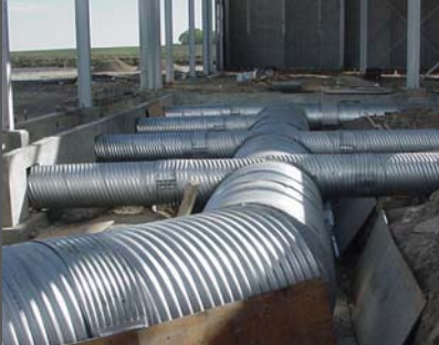
Stormwater Detention Tanks
